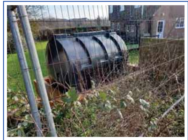
Heating Oil tank in rear garden
