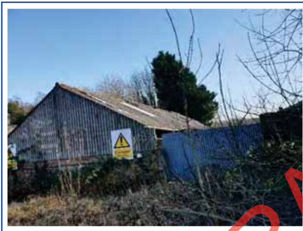
Disused Agricultural Barn labelled with Danger Asbestos
