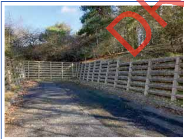
Retaining wall feature within NHS commercial area in the southeast of the site
